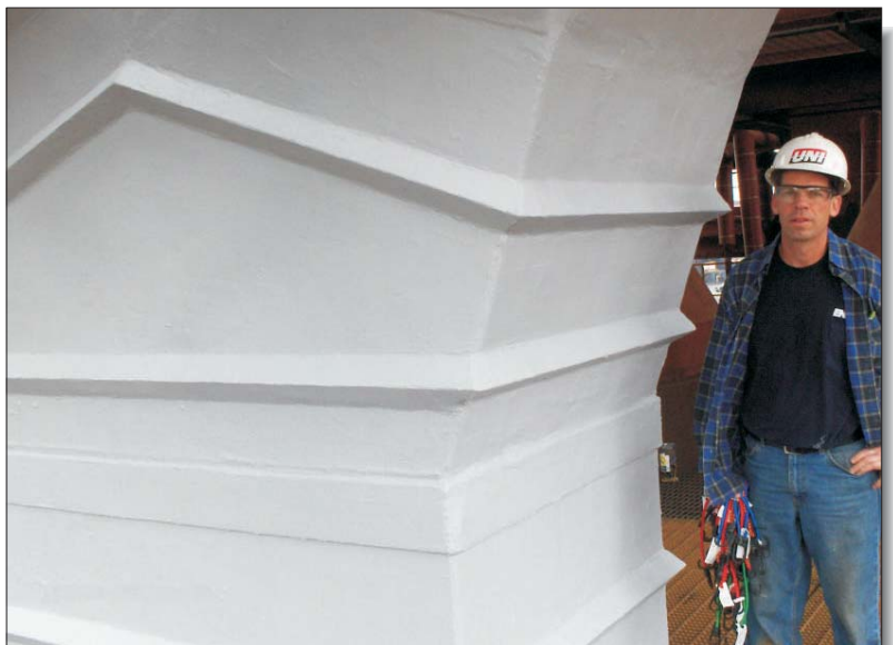
After totally encapsulating the unit in DurAlloy, ENESEAL CR was used to provide optimum corrosion resistance and a uniform look.
