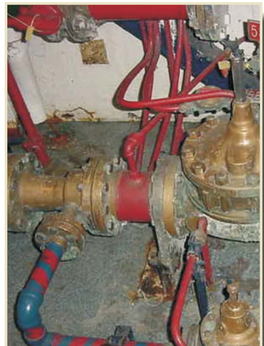
AFFF Station 5 Years ago.
