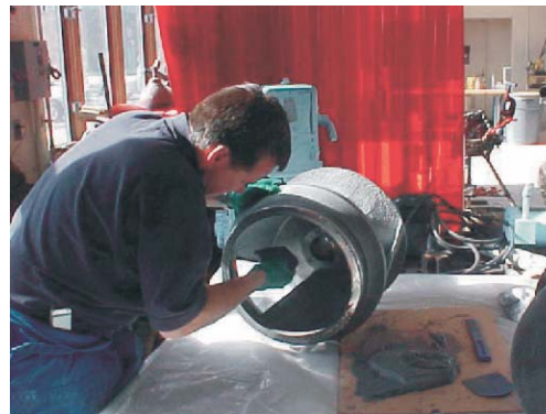
CeramAlloy CP + AC was used to smooth out and rebuild eroded areas of both impellers.
