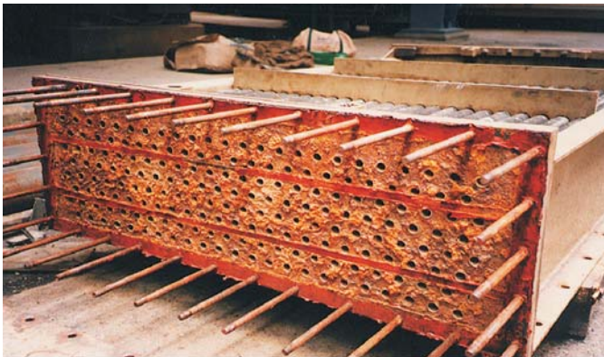
The severely damaged cooler.
