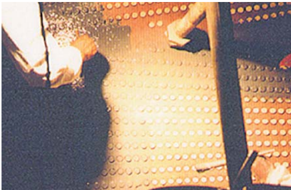
The first coat of CeramAlloy CL+ (Gray) being applied to one of the tubesheets.
