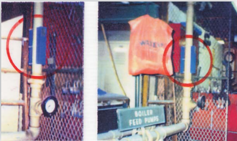
ENEFLOW 5000's installed on boiler feed line.
